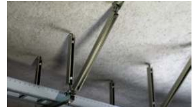
TOLCO seismic bracing
