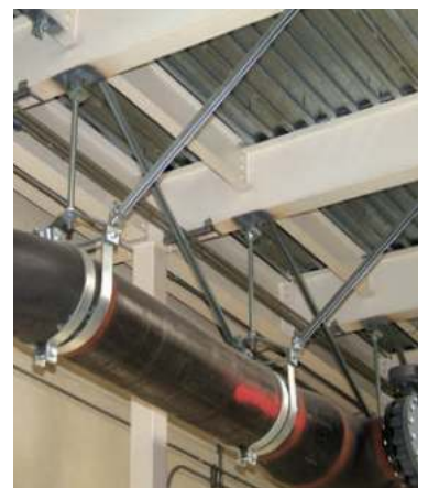
TOLCO seismic bracing
