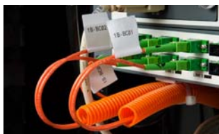
Fiber Optic Cable Markers
